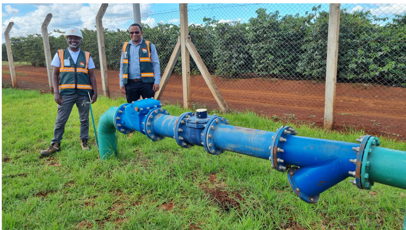
Proud engineers at the pumping station
